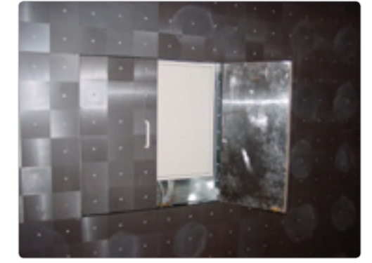
Electrical distribution box access from inside
