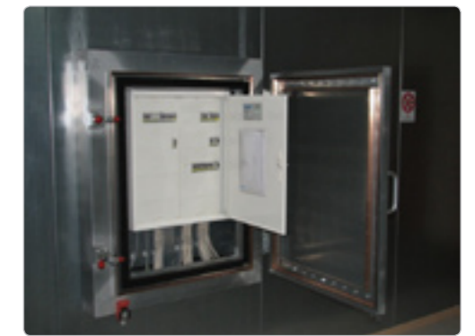
Electrical distribution box access from outside
