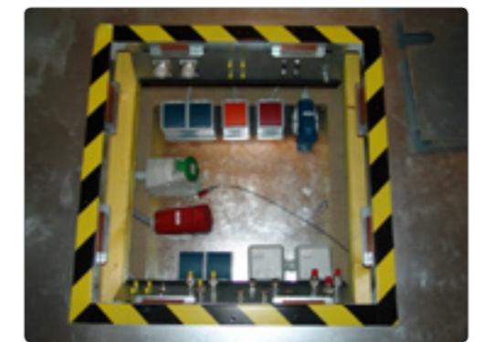
Outlet box in raised floor
